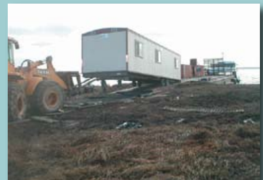
Delivering the new Newtok CVRF office trailer on the new geoblock trail
